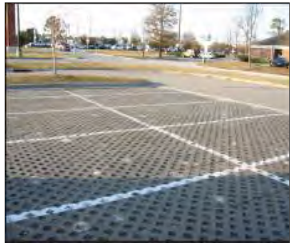
Figure B-30: Example of Open-celled Block Pavers in Overflow Parking Lot (New Hanover County & City of Wilmington, 2008)
