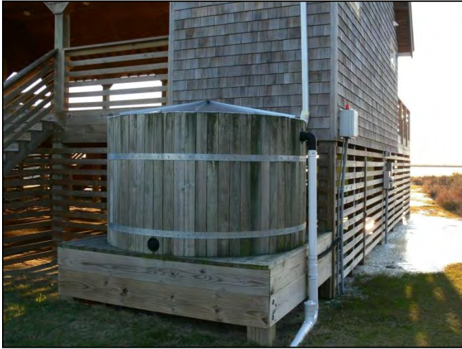
Figure B-33: Cistern for Rainwater Harvesting in Dare County, NC
