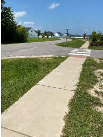
5. Sidewalk section along Gables Place south of Briton Way needs repair.
