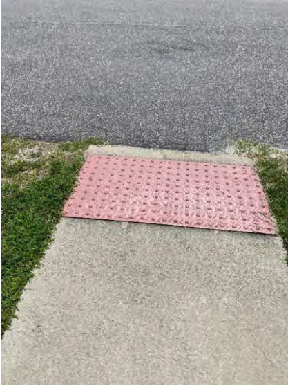
22. Detectable warning mat at Gables Place West.
