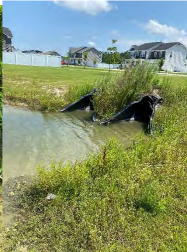
31. Double culverts outletting to control structure (Phase 1 pond).
