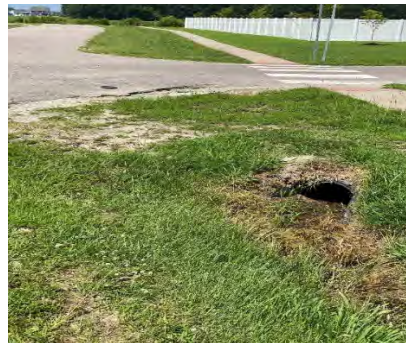
48. Culvert maintenance is needed at Artisan Way/Thayne Drive intersection.
