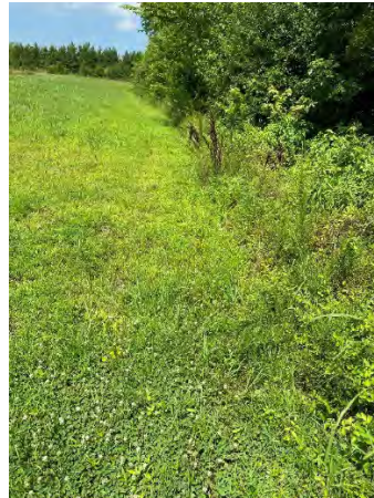
37. Overgrown outlet ditch from Pond 2.
