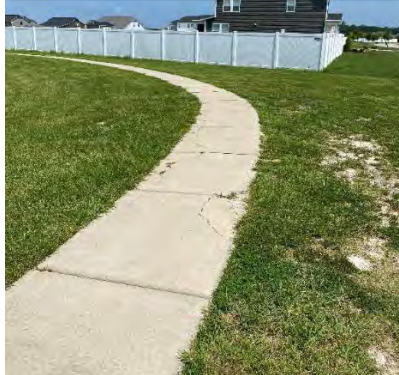
14. Sidewalk behind Lot 22 needs repair.
