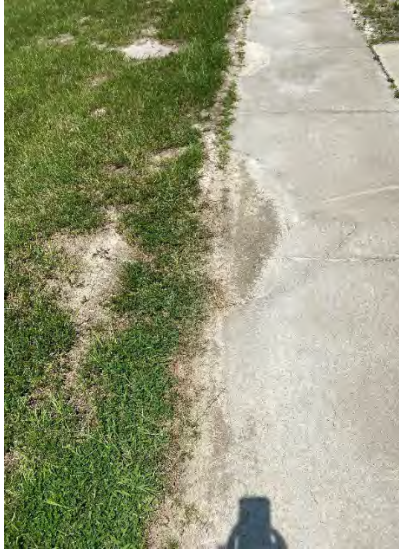
11. Sidewalk section behind Lot 31 needs repair.
