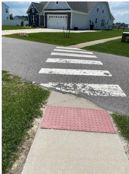
21. Crossing at Gables Way by Phase 1 pond (concrete repair needed).
