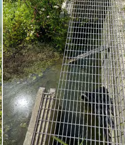
29. Outlet control structure at Phase 1 pond.
