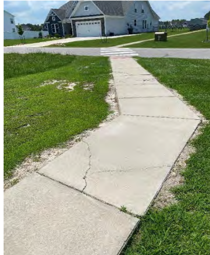
9. Sidewalk in common area across Gables Place from Lot 51 needs repair.
