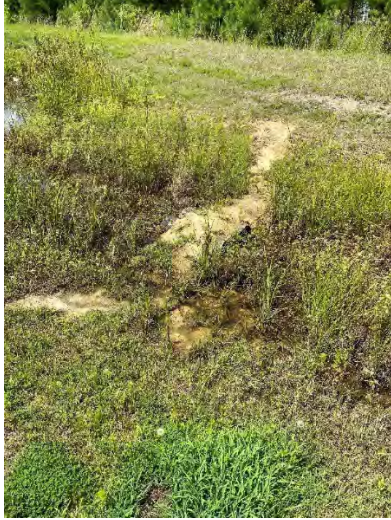
39. Obstruction to flow from Pond 2 outlet structure should be
