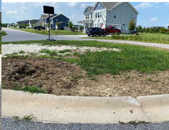
54. Cul-de-sac at end of Gables Place – curb needs minor repair. (Note: Island is a community association responsibility.)
