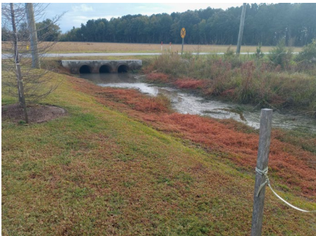
Photo #46 – Outlet Ditch and Culverts under Baxter Lane, Facing South appears to need some vegetation removal
