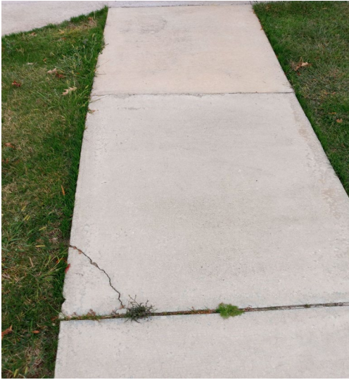
Photo #16 - Sidewalk in front of Lot 21, Facing North with cracked corner
