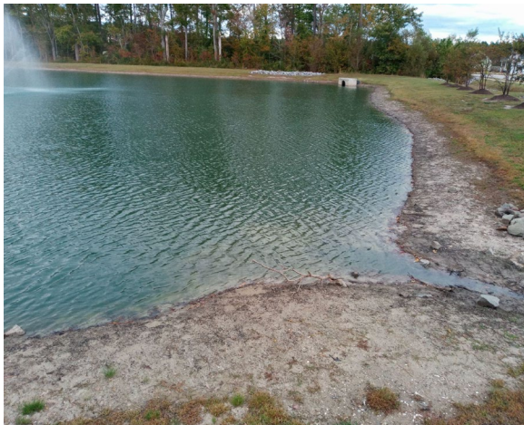
Photo #47 - East side of Stormwater BMP 1, Facing North. Some additional stabilization appears to me needed here.
