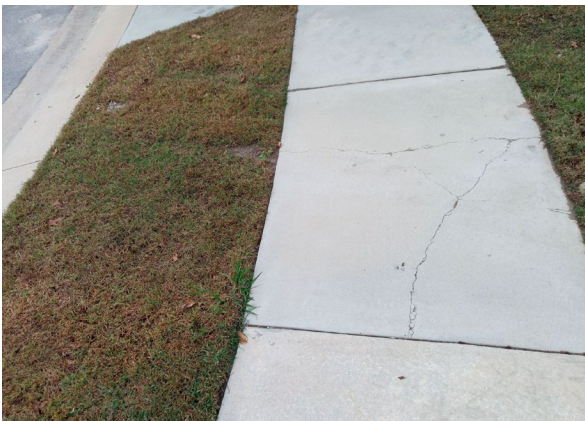
Photo #22 – Cracked sidewalk in front of Lot 10, Facing South
