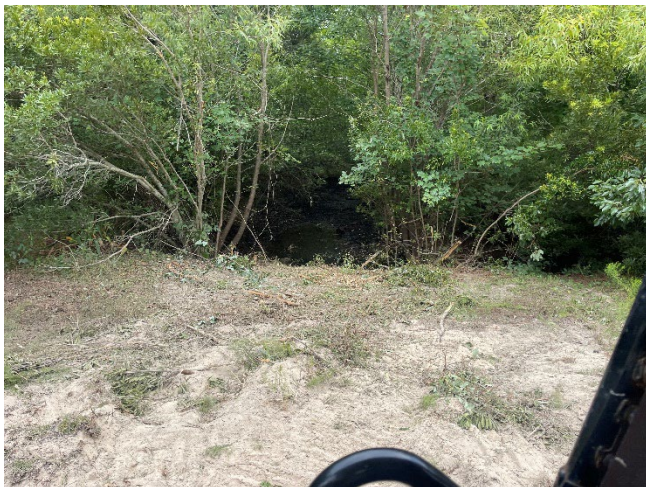
Culvert and swale at Sandfiddler Road cul-de-sac were opened up and made functional.
