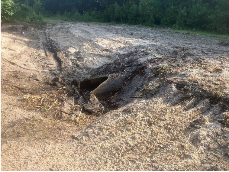
Buried culvert at Rock Lane was exposed and cleaned, and connecting roadway swale was regraded.
