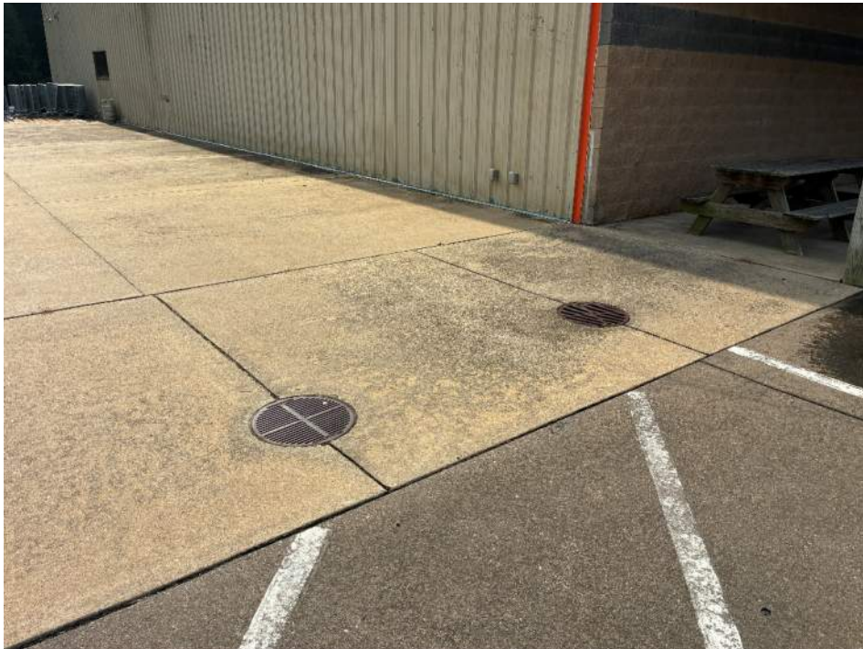
Photo 16 – Two of four drop inlets east of the main treatment area.
