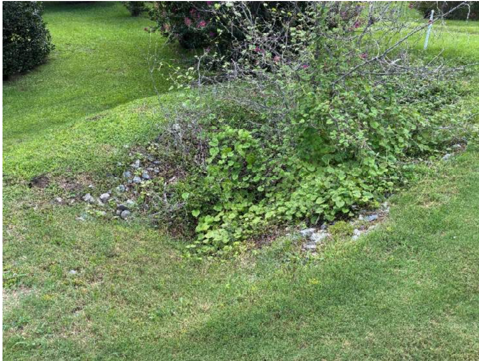
Photo 15 – Culvert and riprap south of the overflow device covered in vegetative growth.
