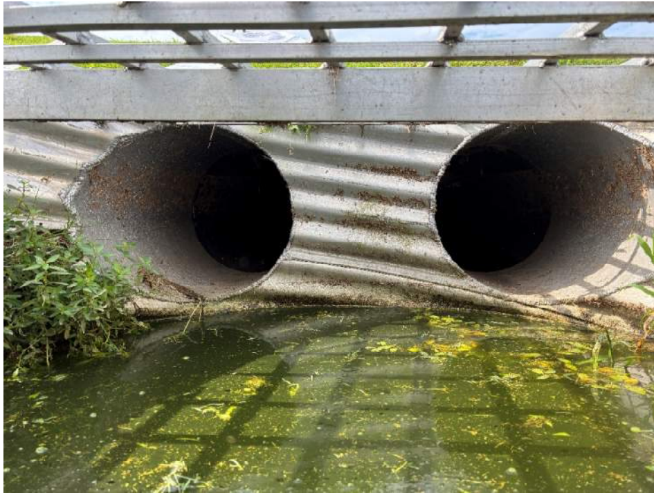
Photo 13 – View within the overflow device, facing south.
