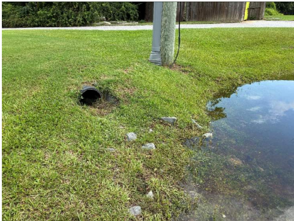
Photo 2 – Riprap and 15" culvert inlet on the north side of the main treatment area with sedimentation.
