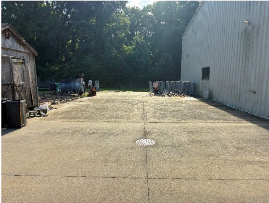
Photo 17 – Two of four easternmost drop inlets east of the main treatment area.
