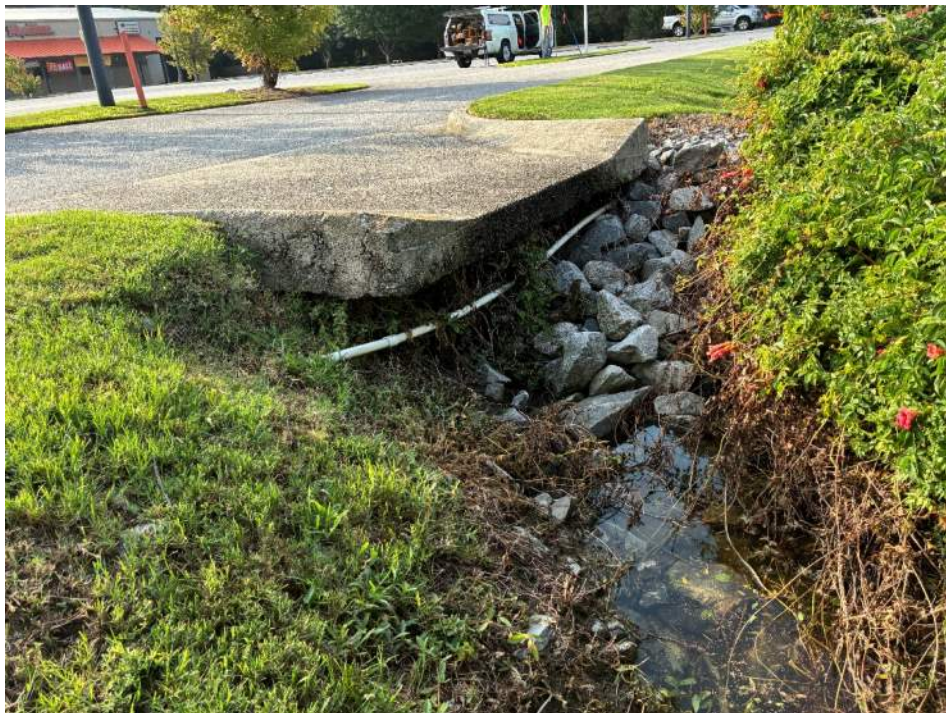
Photo 8 – Bank erosion beneath the concrete flume.
