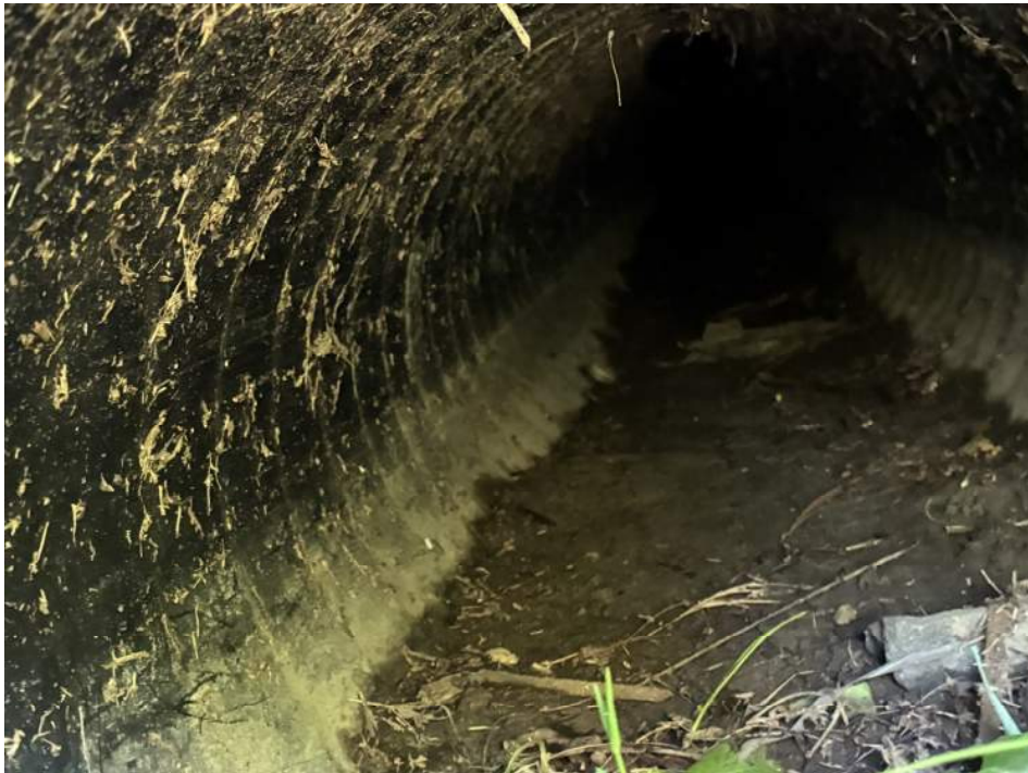
Photo 6 – Sedimentation within the culvert seen in Photo 5.
