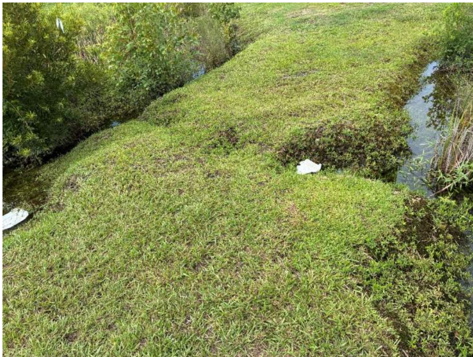
Photo 10 – View of erosion along the forebay berm.
