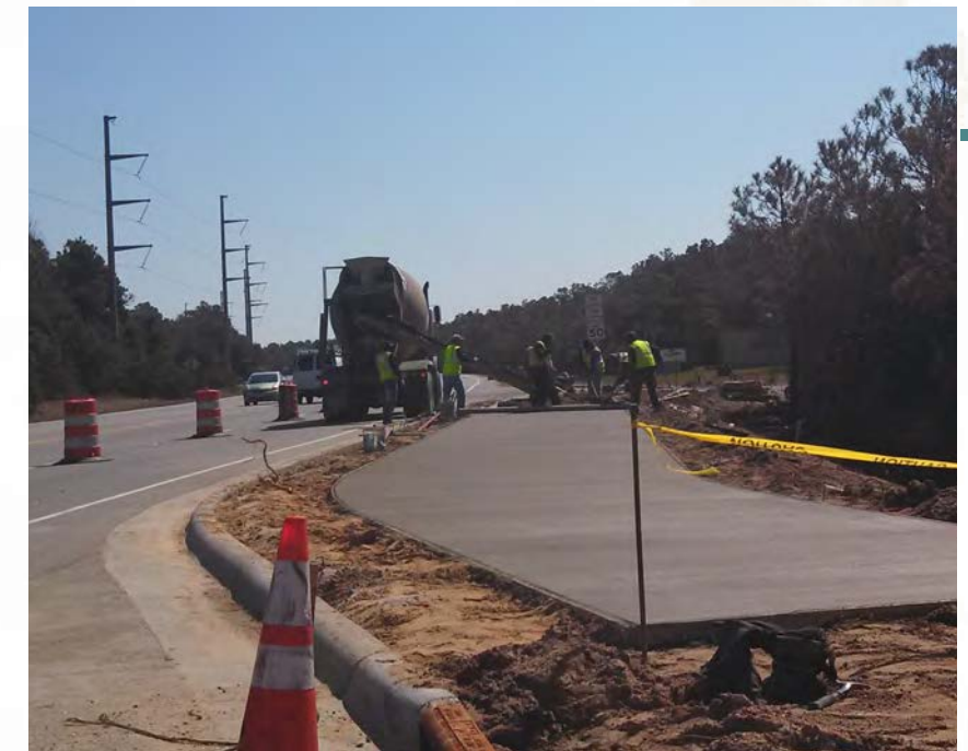
Multi-use sidepaths are increasing in mileage across the Outer Banks such as this one being constructed along NC 158 in Nags Head in 2013. Most bicyclists prefer a separated facility which is also safer than bicycling in the road.
