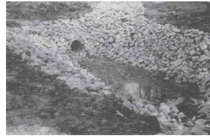
Figure 6.41a Riprap outlet stabilization structure prevents erosion by reducing velocity of concentrated flow.
