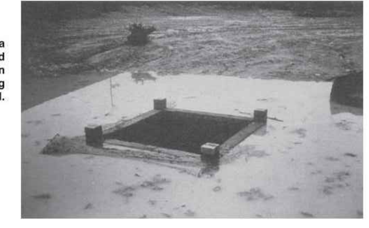
Figure 6.50a Excavation around inlet creates an effective settling pool.
