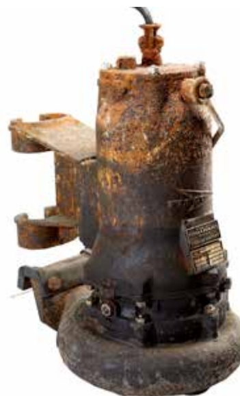
The effects of general corrosion on a wastewater pump that is still functioning after 50 years of use.
