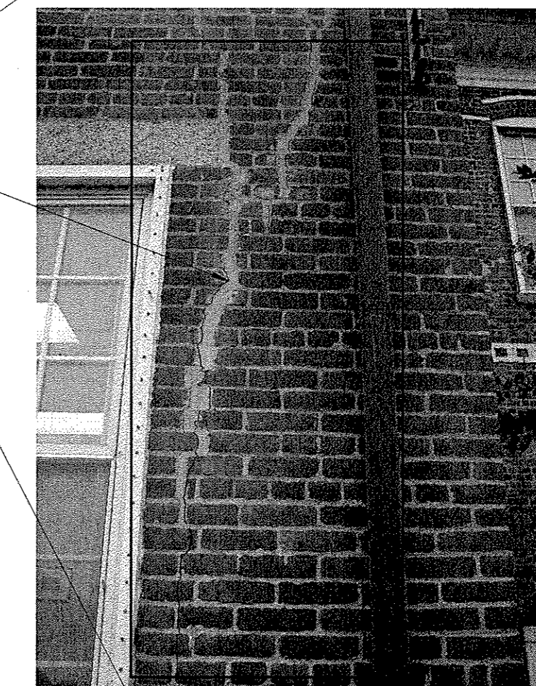
NORTHEAST CORNER OF HISTORIC COURTHOUSE WHERE MASONRY REPAIRS ARE REQUIRED
