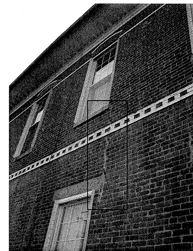
CUT OUT AND REPLACE BROKEN BRICK THIS AREA AS SPECIFIED
