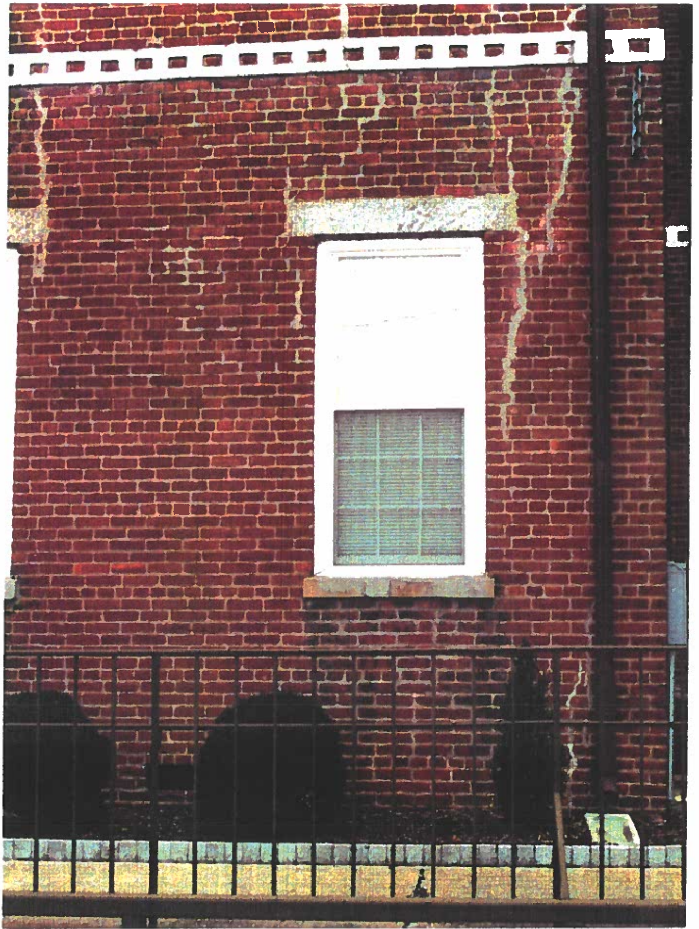
MASONRY CONDITIONS AT EAST ELEVATION
